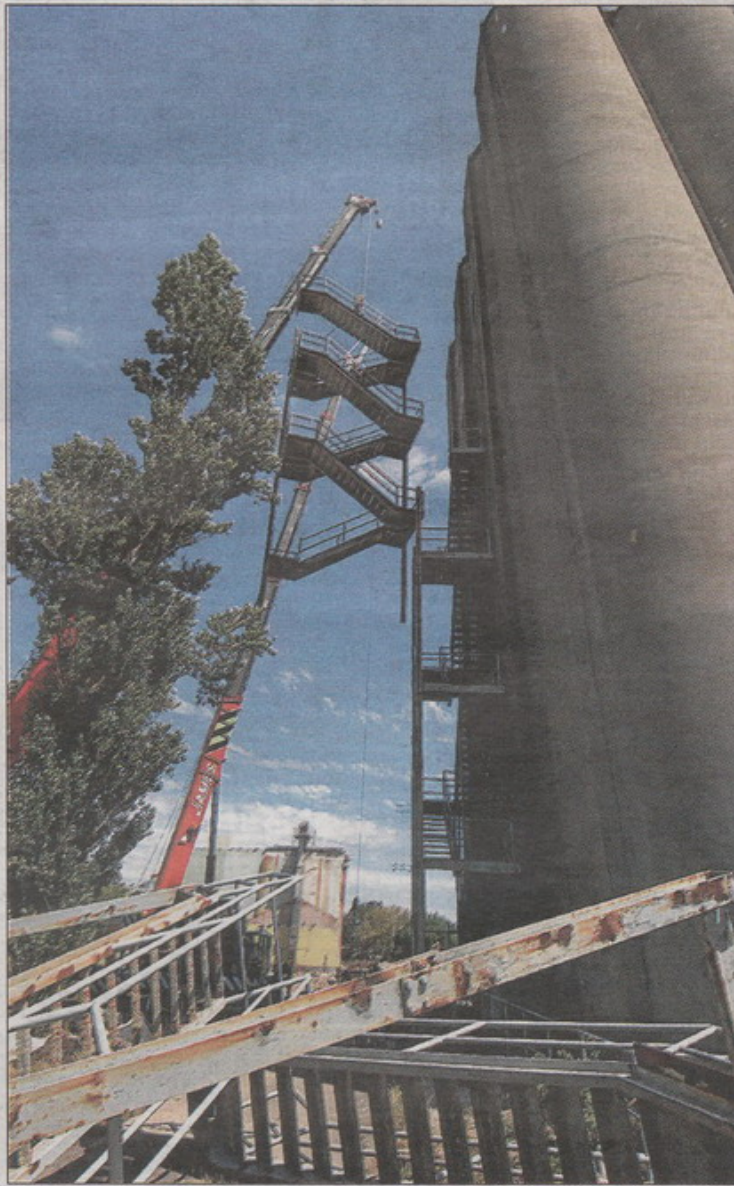
COMING DOWN: A crane removes the external stairs from the old Joe White Maltings silos in Gregory St yesterday. Picture: Jeremy Bannister 300108/06A
